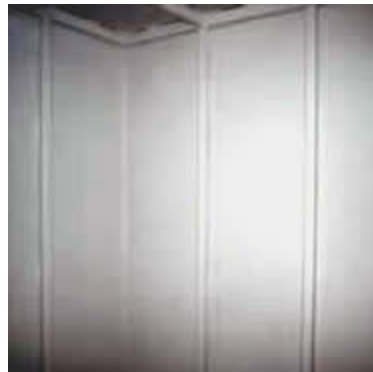
Inside Tubular Frame
